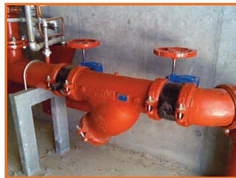
Edipower 800 – Power Plant, Italy
