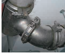
SS 304 potable water line
